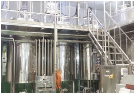
2,000L Mixing Tank
