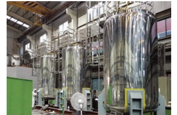
30m 3 Storage Tank
